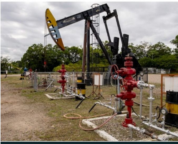
Wellhead and production site
